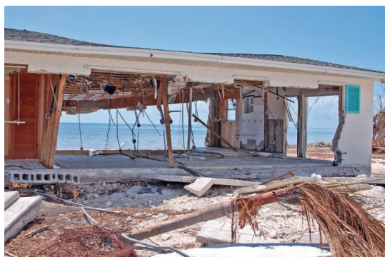
Figure 3-6: House constructed at grade where the masonry walls parallel to the shoreline were destroyed (Big Pine Key)
