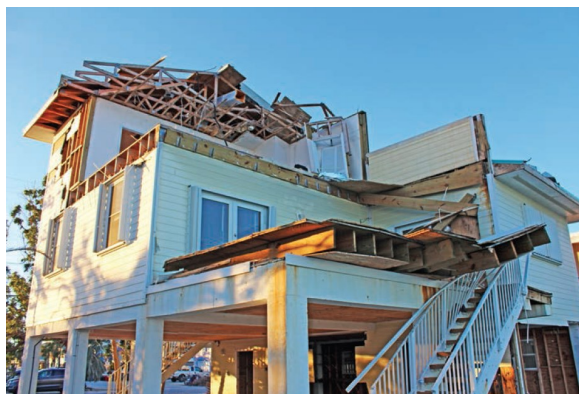
Figure 4-6: House with roof structure loss and collapse of the second floor exterior wall and adjacent deck (EWS=113 mph; EDWS=180 mph) (Ramrod Key)
